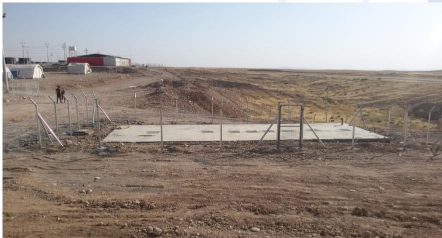
Figure 5: Finished DEWATS fenced in
