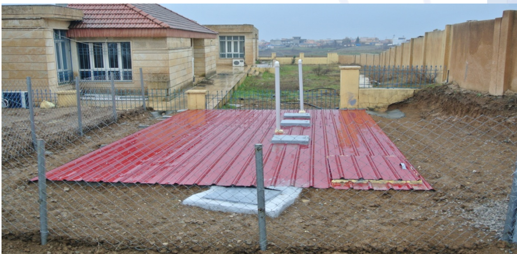
Figure 4: Because of the rainy season we prepared an iron shed with drainage for rainwater
