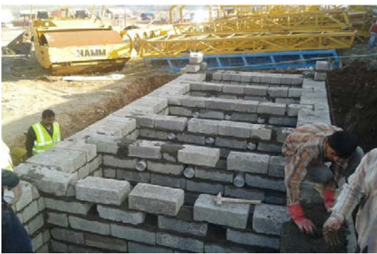
Figure 1: The procedure of casting the concrete of the foundation then starting the solid block wall, installation of 4" pipe and covering the external faces of the wall with cement plaster.
