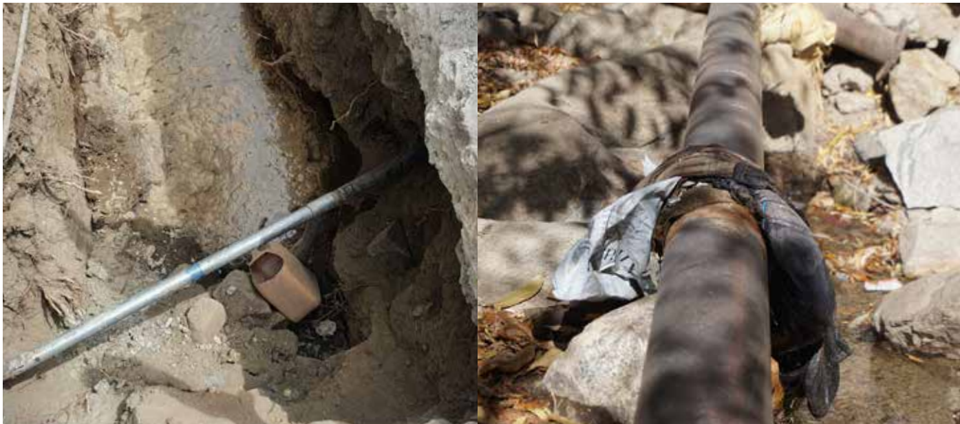
(Uninsulated, above ground broken pipes)
